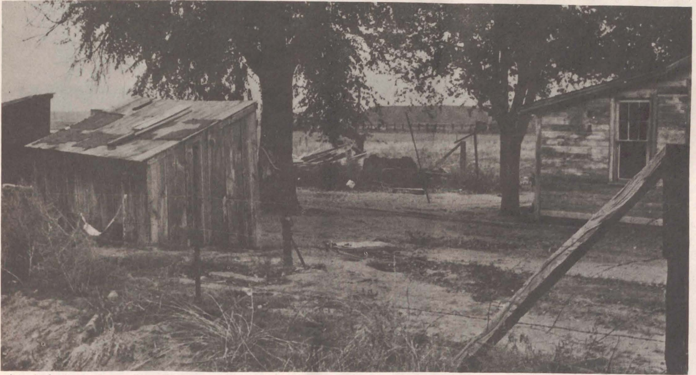
A typical migrant house. Note the outhouse and outside hand pump. The dump, in background, will attract insects. There are no windows.
